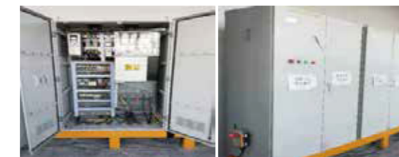
Layout in crane and trolley cabinets
